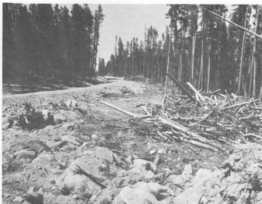
FIGURE 4. Trucking road on moraine. Swath cut for road averages 30 m in width for a roadbed of only 5 m near Mosquito Lake. Teton Forest, Wyoming.
